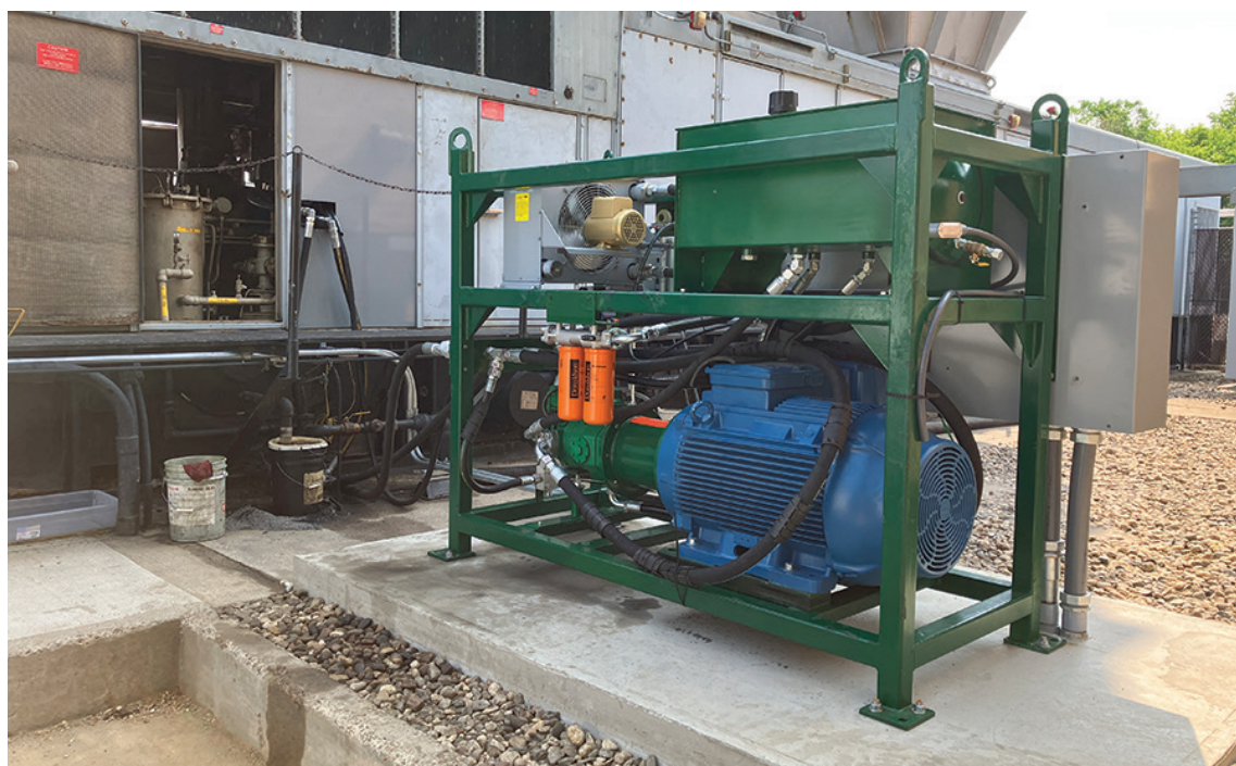
The new "skid", the electric pump and starting motor that replaced the 1968 Cummins Diesel.
