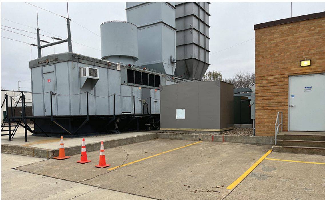
An overall view of Marshall's turbine.
