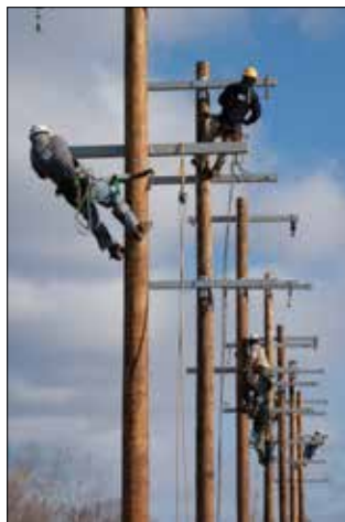
One of four pole lines on the Apprentice side of the rodeo field.
