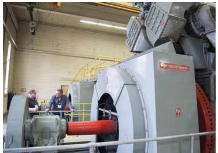
MMUA partners with the League of Minnesota Cities Insurance Trust to develop guidelines for the safe operation of local electric generating plants.
