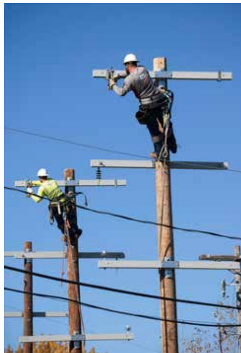
MMUA training (including this scene from the Minnesota Lineworkers Rodeo) helps develop an effective mutual aid response.
