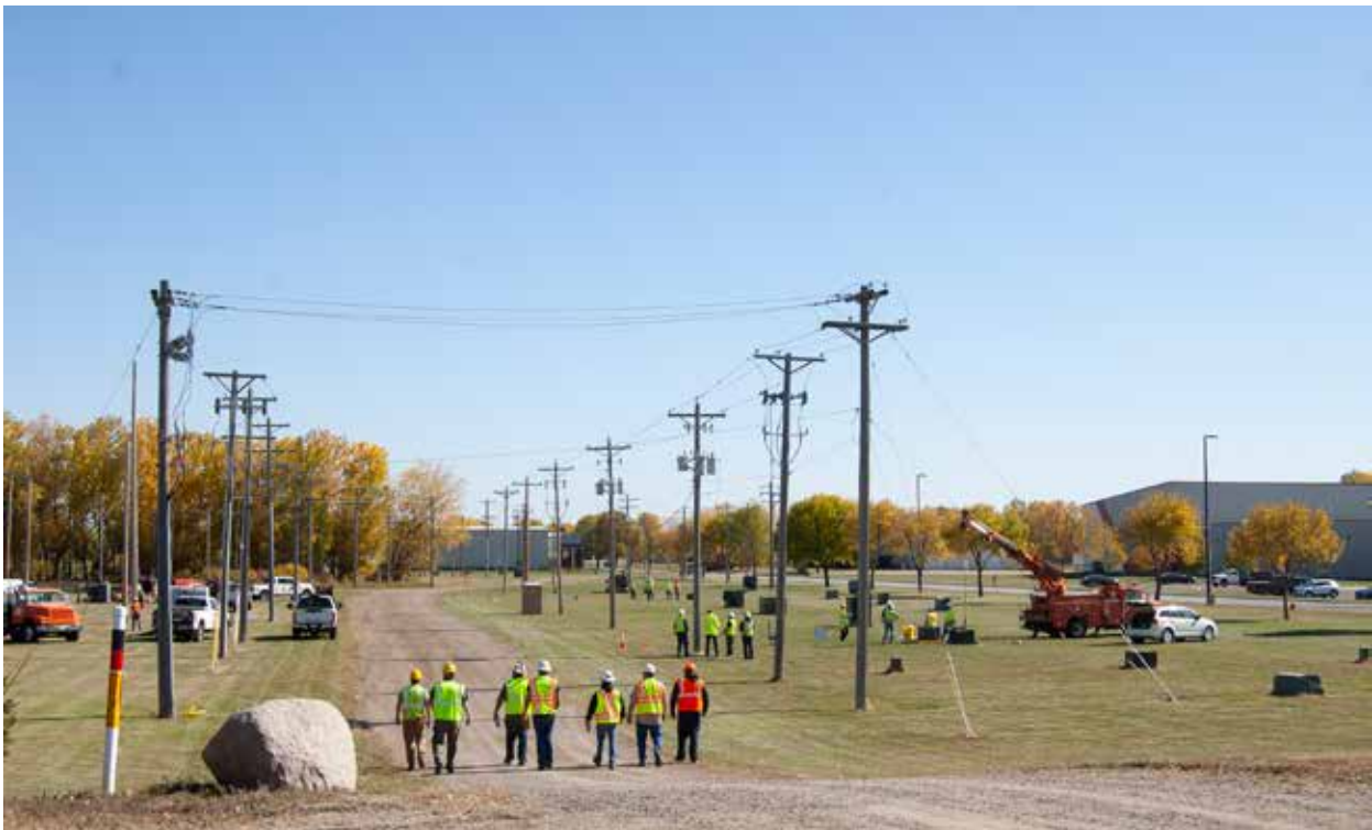
MMUA closed on the purchase of the MMUA Training Center property on March 4, 2020. MMUA began leasing the approximately 18 acre property in 1999 and has made numerous improvements since then. This picture shows a portion of the property.
