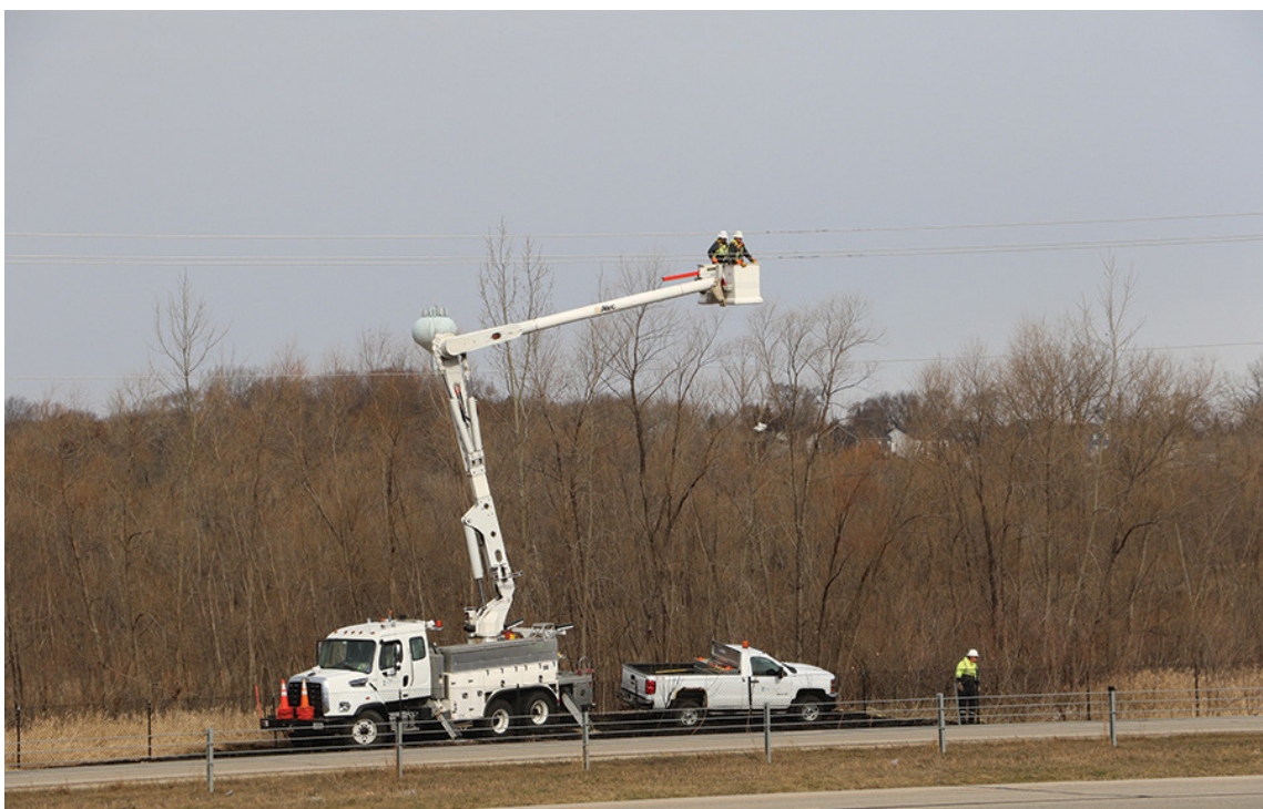
RPU crews inspect the affected power lines on the morning of March 21, the day after the hot air balloon crash. (Photo courtesy of Rochester Public Utilities.)
