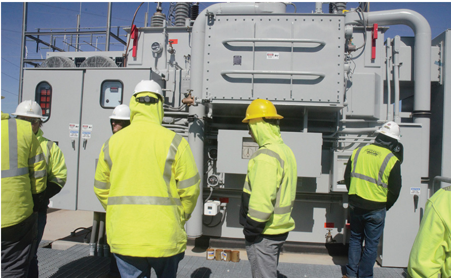
Attendees toured the West Shakopee substation.
