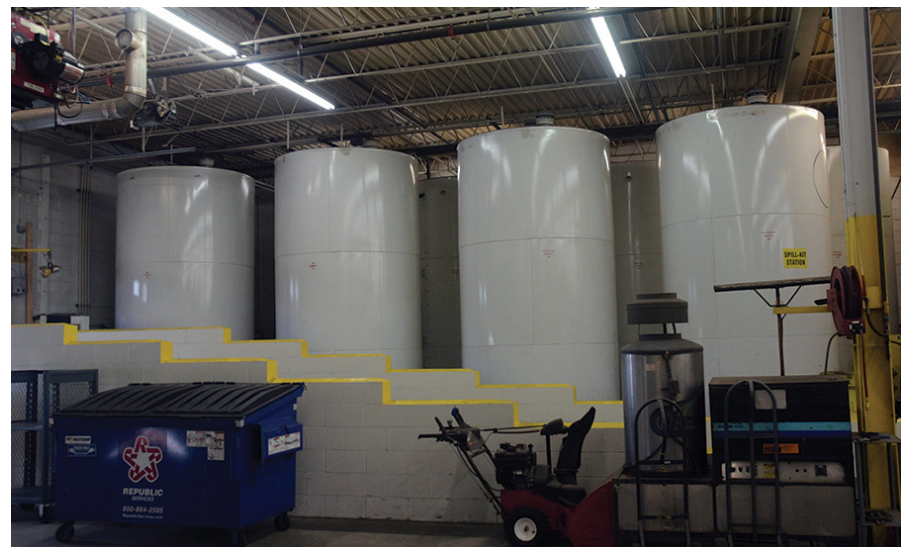
The giant tanks hold mineral oil for use in rebuilt transformers.
